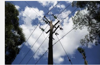
Electricity lines near sawmills
